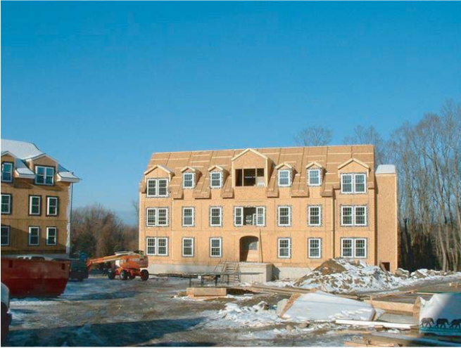
Construction on the buildings was quick and efficient thanks to the prefabrication of the panels and other materials supplied by Panels Pros.
