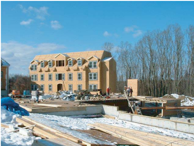
The expansive job site allowed multiple processes of the building to be performed at the same time.
